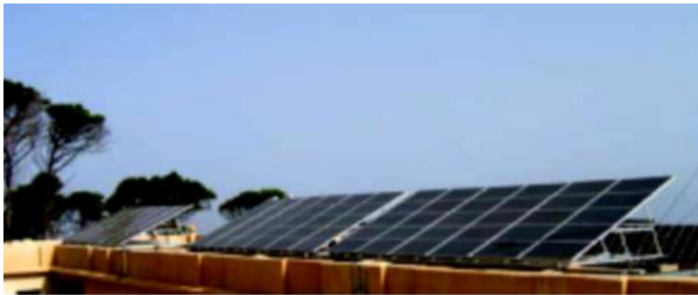
Figure 2. Roof small grid connected PV plant in Algiers, Algeria. [3]
